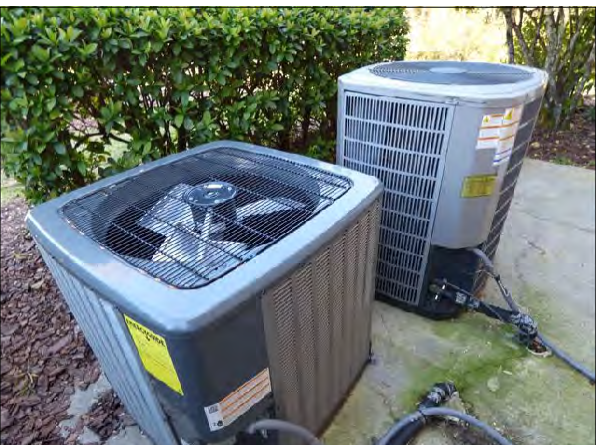
Nature Center HVAC
