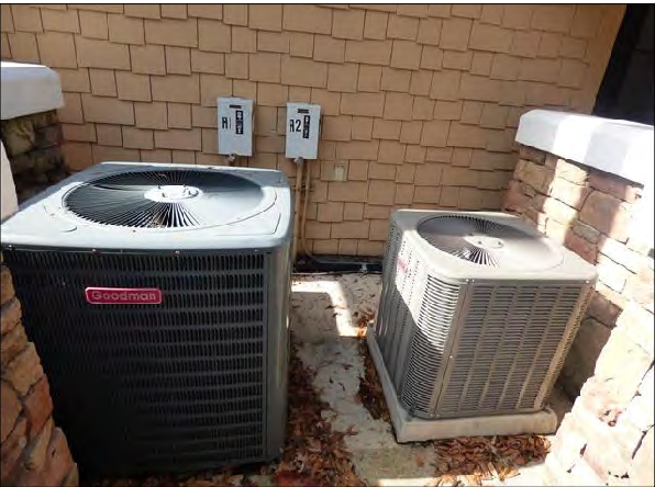
Activity Center HVAC
