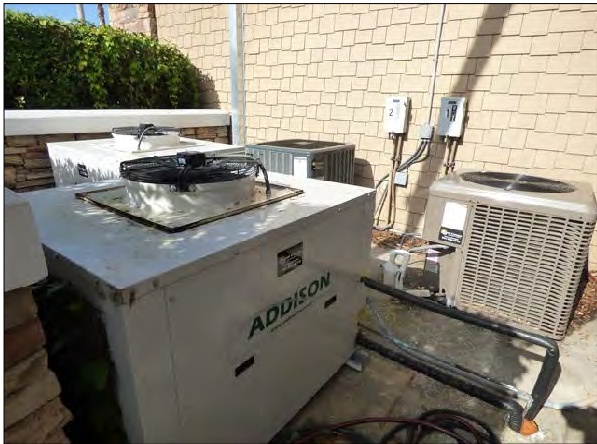
Fitness Center HVAC
